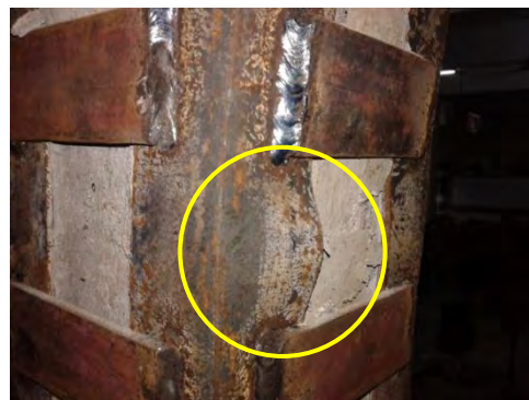
Figure 5.12 Buckling of steel angles and concrete spalling in between strips with an eccentricity of 37.5mm
