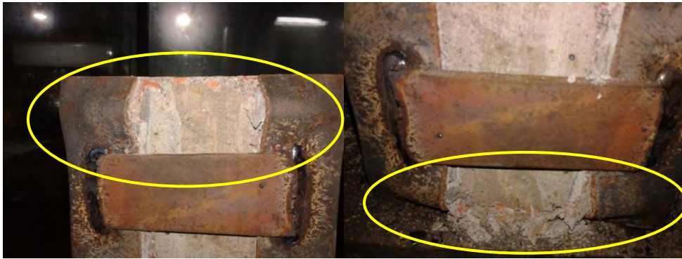
Figure 5.7 Steel angles buckling at (a) Top and (b) Bottom of strengthened RC column under concentric loads
