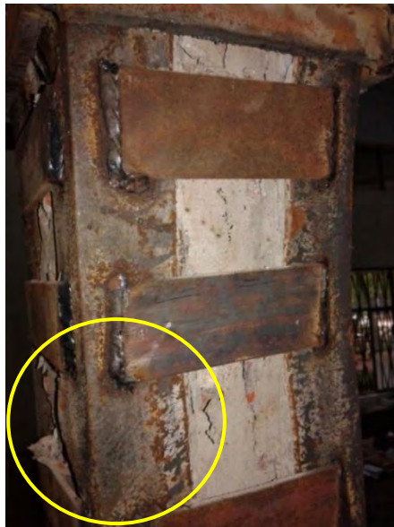
Figure 5.10 Buckling of steel angles and concrete crushing in between strips with eccentricity of 15mm
