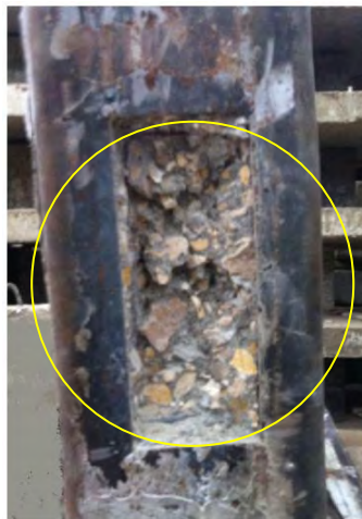
Figure 2.6 Failure of jacketed column by concrete splitting
