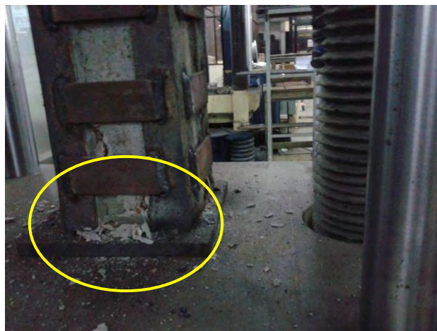
Figure 5.8 Concrete splitting of strengthened RC column at bottom under concentric loads
