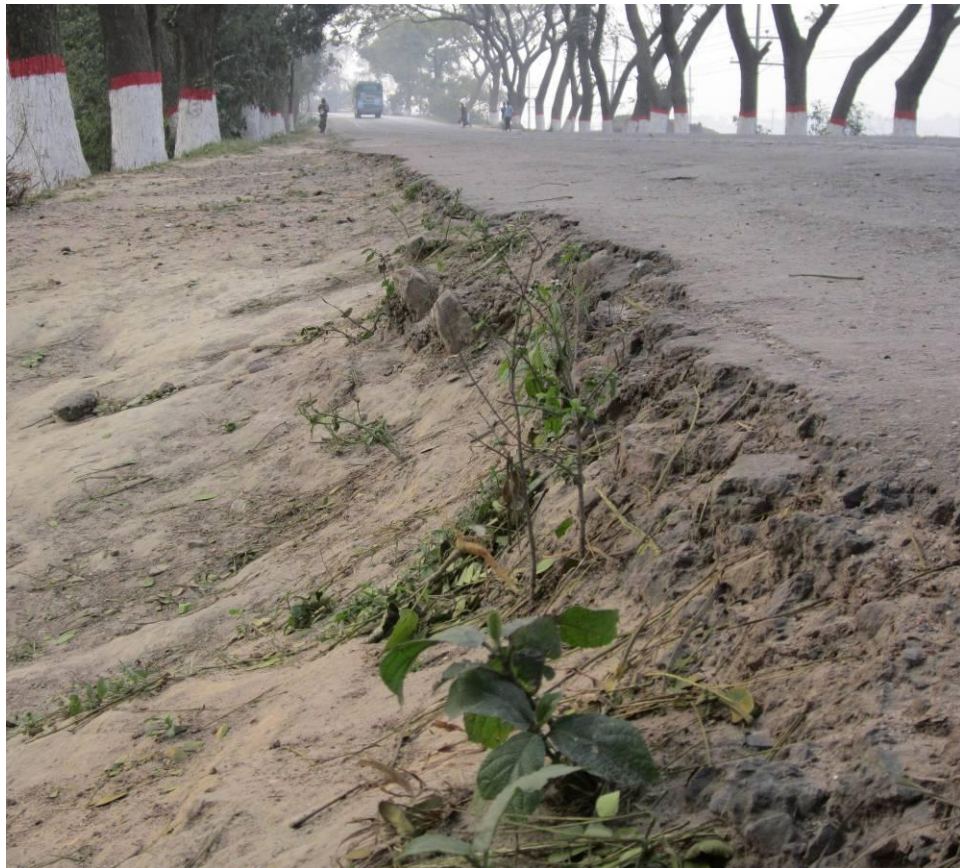
Figure 3.2: Shoulder Damage due to Rutting of Soft Soil
