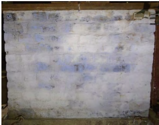
Figure 4.17 Initial Crack (Flexure) Pattern of Specimen C-1/2
