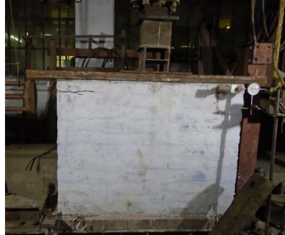
Figure 4.25 2 nd Cracks (Shear) Patterns of Specimen C-3/4
