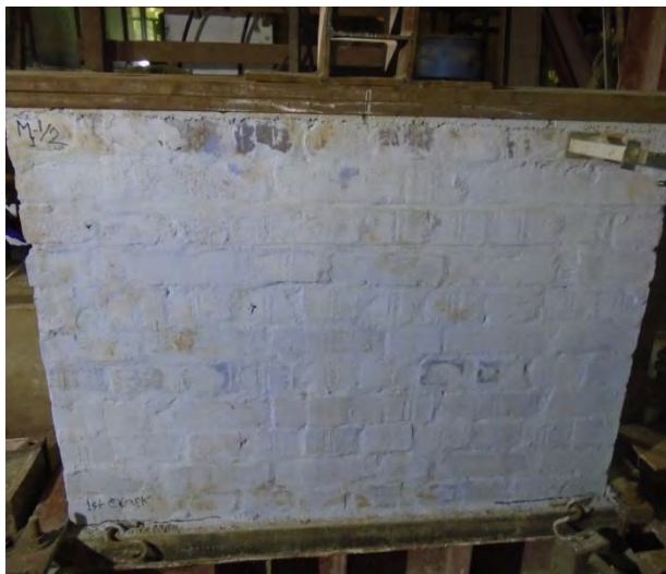
Figure 4.34 Initial Crack (Flexure) Patterns at Specimen M1-1/2
