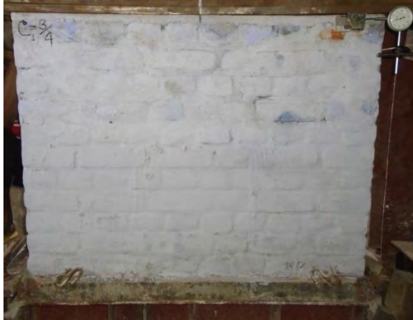
Figure 4.28 Initial Crack (Flexure) Patterns at Specimen C1-3/4
