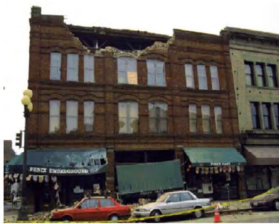
(d) Nisqually earthquake February 28, 2001
