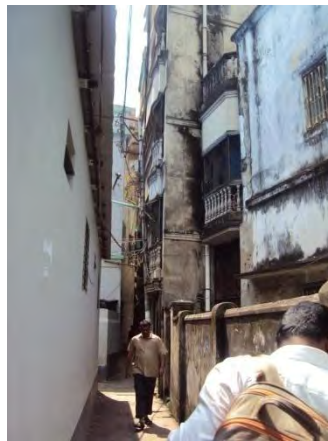
Figure 4.59: Inadequate penetration of sunlight
