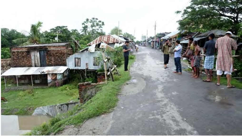
Polder 17/1, 1-Vent 1.50X1.80 regulator broken
