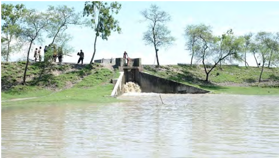
Polder 17/1, 1-Vent 1.50X1.80 regulator water is draining out
