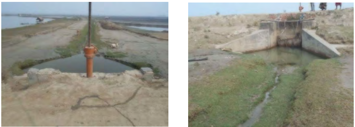
Figure 4.2: Present condition of DS-5 in polder 17/1(C/S at figure-a and R/S at figure-b)
