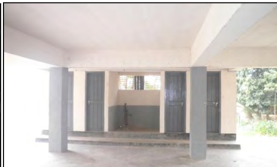
Photo 3.15: MPCS made by CARITAS in Dhankhali Union (Ground Floor Toilet and Tube-well)
