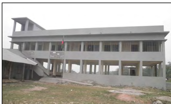
Photo 3.8: One stair of MPCS without ramp made by LGED (Source: Field Visit, February 2013)
