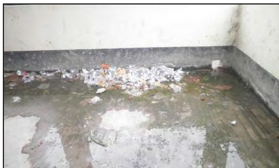
Photo 4.24: Inside of MPCS in Lalua Union Used as to Keep Waste and Garbage.
