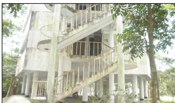
Photo 3.9: Three Storied Building of MPCS Made by Grameen Bank in Nilganj Union
