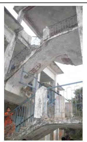
Photo 5.10: Damaged plastering of stair of MPCs in Lalua Union
