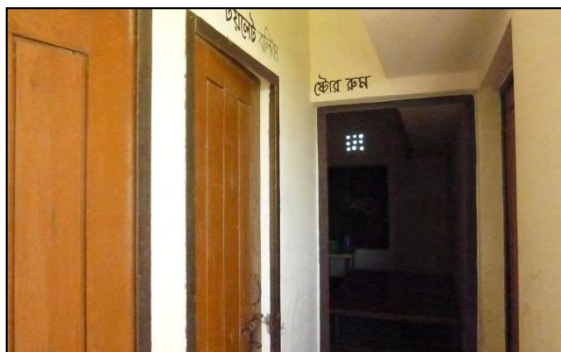
Photo 3.22: Small Store Room of MPCS in Mithaganj Union (Source: Field Visit, February 2013)
