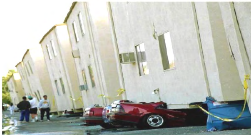
Figure 3.5: Soft storey failure
