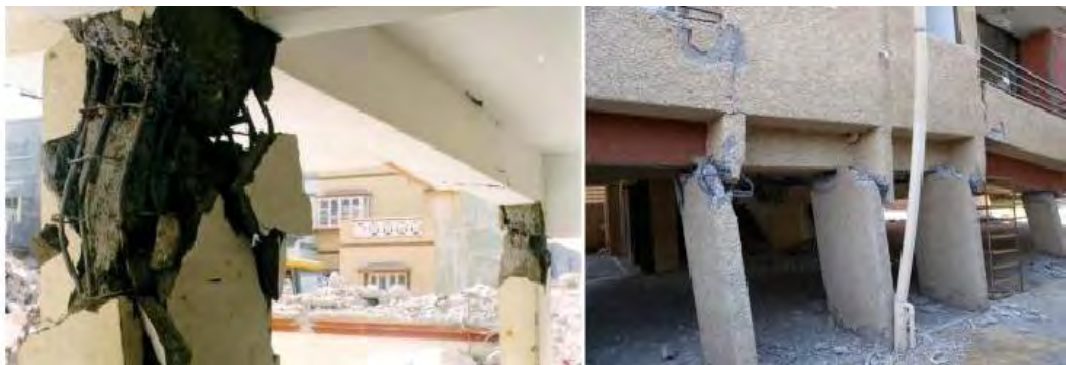
Figure 1.4: Damages in columns during earthquake
