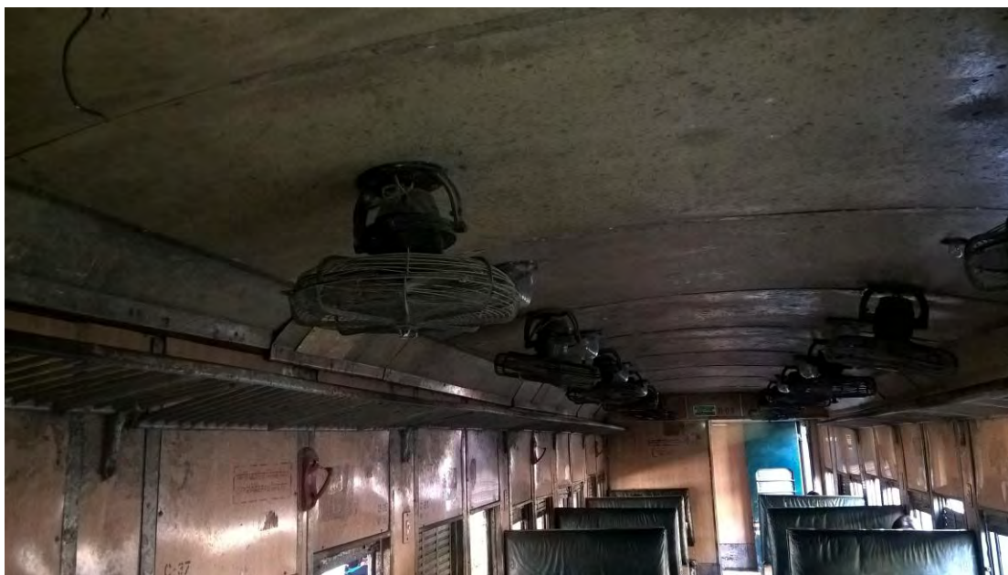
Figure 4.14 Air ventilation system of Intercity Train
