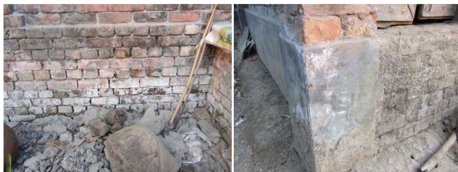
Figure 5.14: Salt patches and damage of the bricks and plasters
