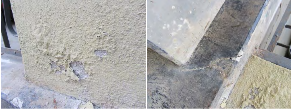
Figure 5.15: Blistering in plaster and crack effects due to surge water of cyclone SIDR
