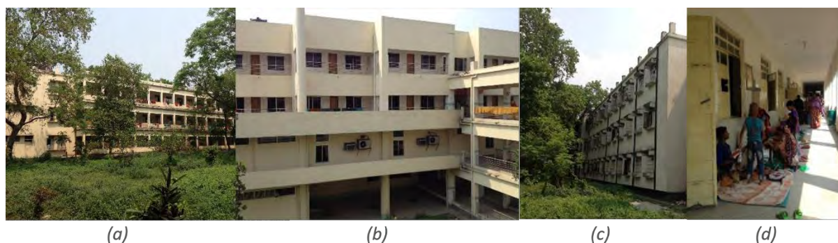
Figure 3.2 Envelope of Hospital building from field survey, (a) surgery inpatient room (b) cardiology inpatient room (c) neurosurgery inpatient room (d) corridor of surgery inpatient room - Rajshahi Medical College, Rajshahi.
