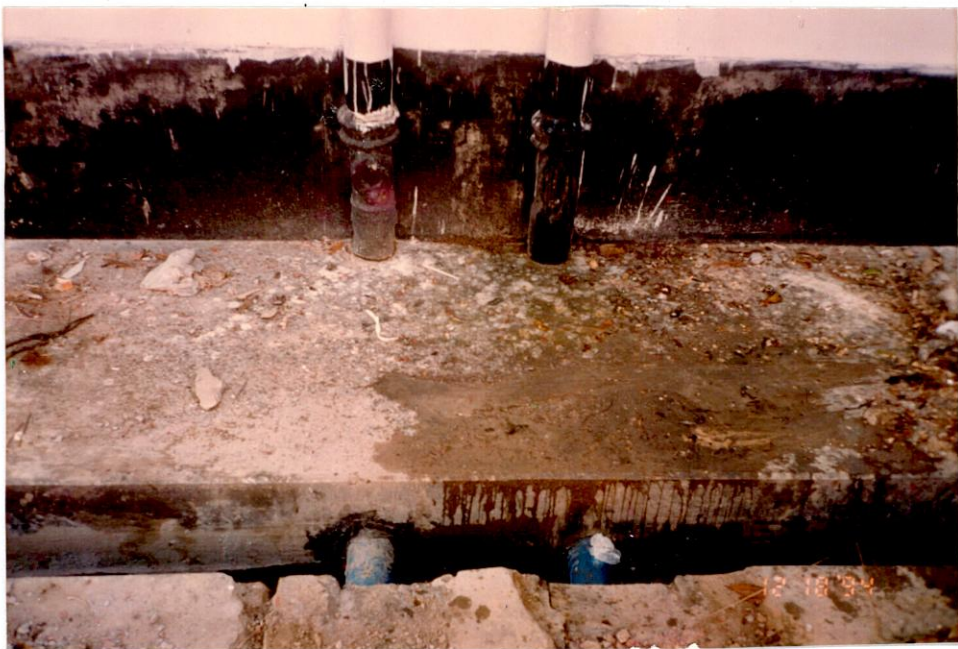
Plate B-2 : Blue pipes showing kitchen and bathroom wastewater connection to septic tank.
