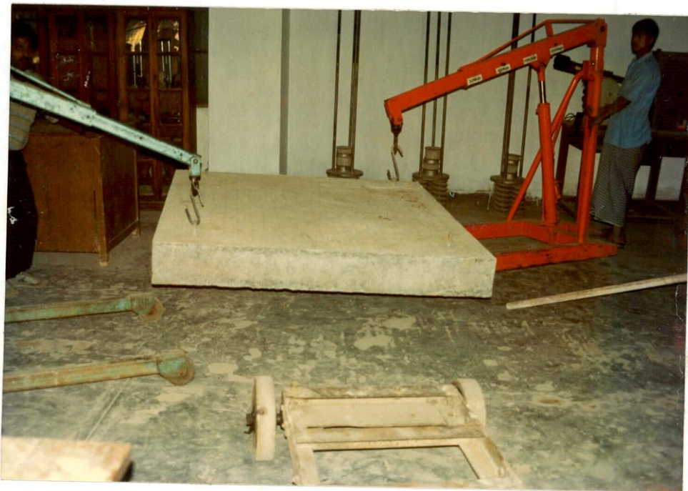
Figure C-4 Lifting of slab with two cranes for placement in the test rig.
