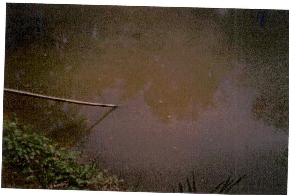
Plate-4.1: Leakage in Unsupported Intake Pipe at Kachua, Chandpur
