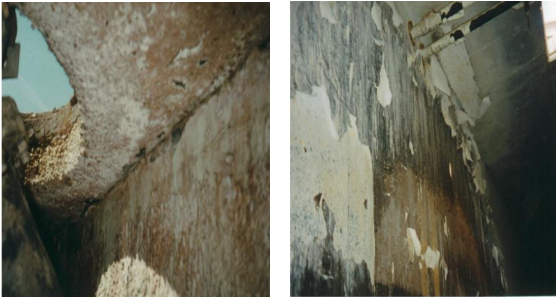
Figure 2.6: Biogenic Corrosion / Vapor Phase due to Sulfide Attack on Concrete
