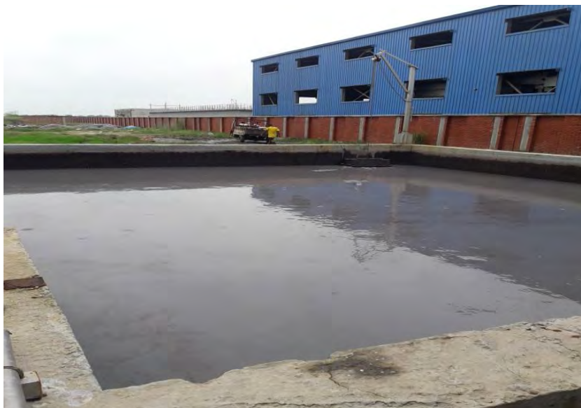
Fig. 4.1 Effluent treatment, tannery estate, Savar, (Author)
