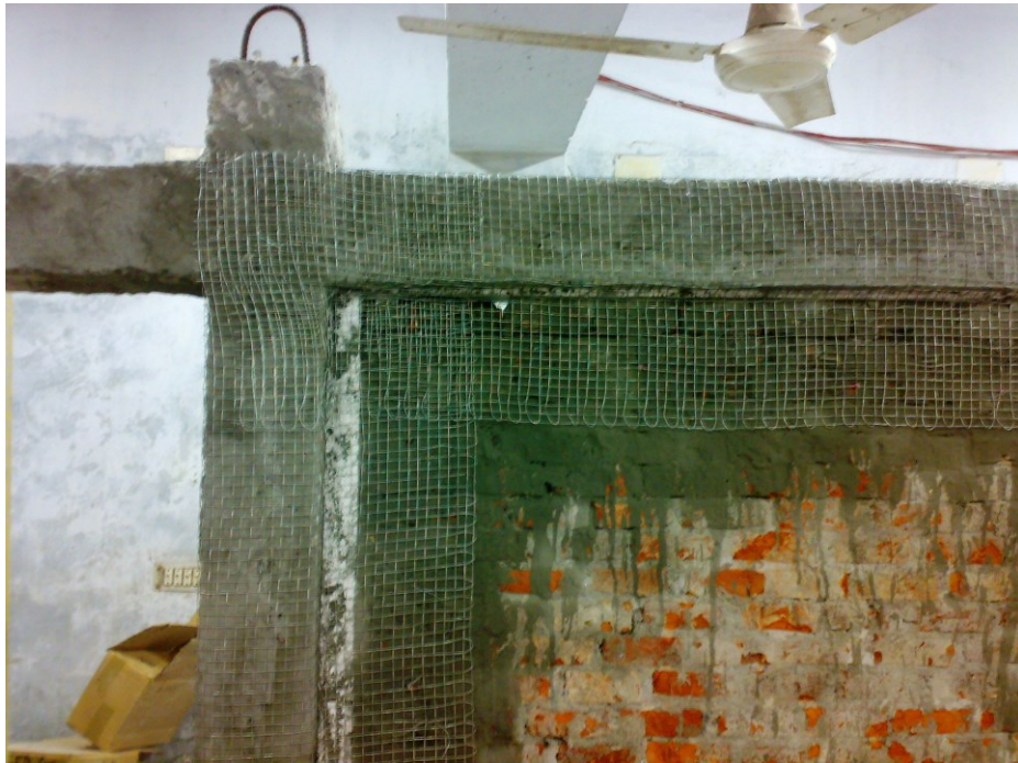
Figure 3.30 Close up view of wire mesh wrapping around the RC frame and infill-RC frame interface for the isolated infilled RC frames
