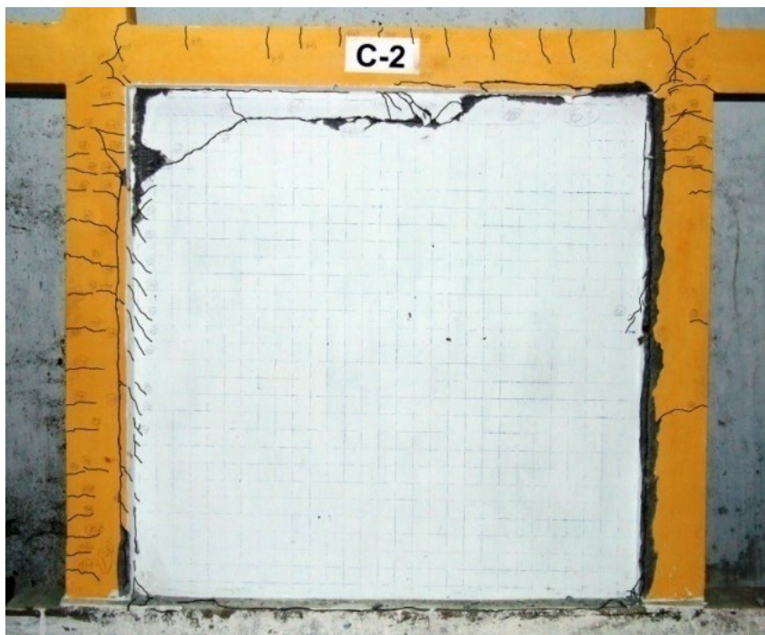
Figure 4.13(b) Crack patterns at maximum lateral load in isolated infilled RC frame specimen C 2
