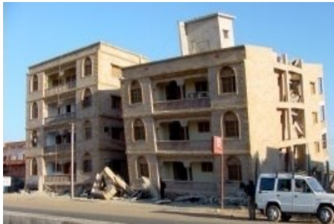
Figure 1.3 Bhuj earthquake in 2001 (India) (Source: NICEE)
