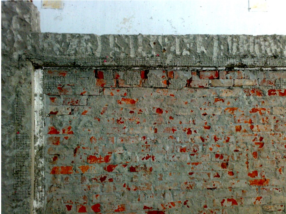
Figure 3.27 Shear sliding, mortar bed joint failure and corner crushing of the isolated in-fill have been identified clearly after chipping of the plasters
