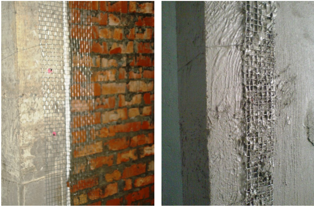
Figure 3.21 Application of sand cement mortars on the specimen surface and the wire mesh fastened along the infill-RC column interface
