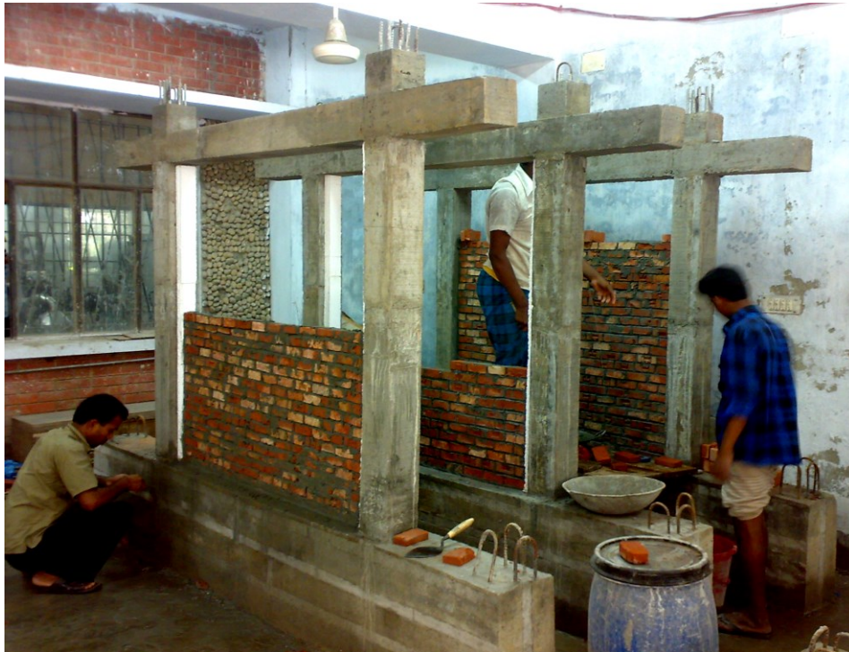
Figure 3.17 Construction of brick infills in specimens C1, C2 and A1 (from front)
