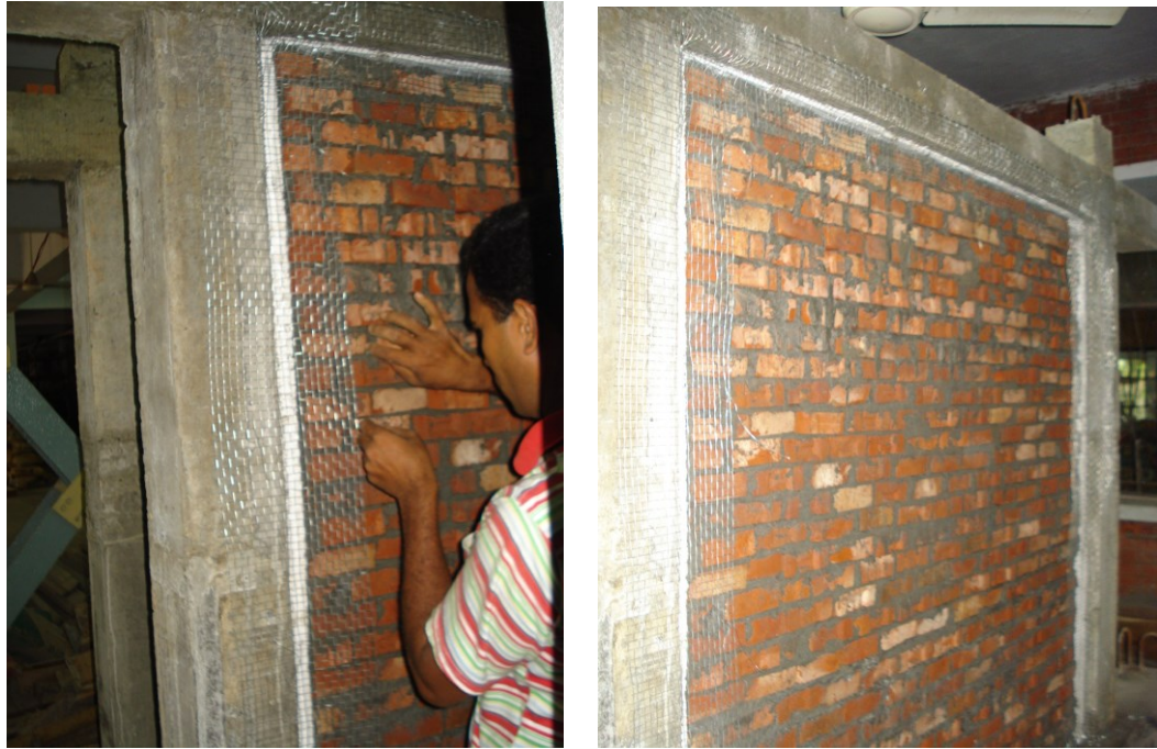
Figure 3.20 Application of wire mesh with GI wire and nails along the surface area of the infill-RC column interface
