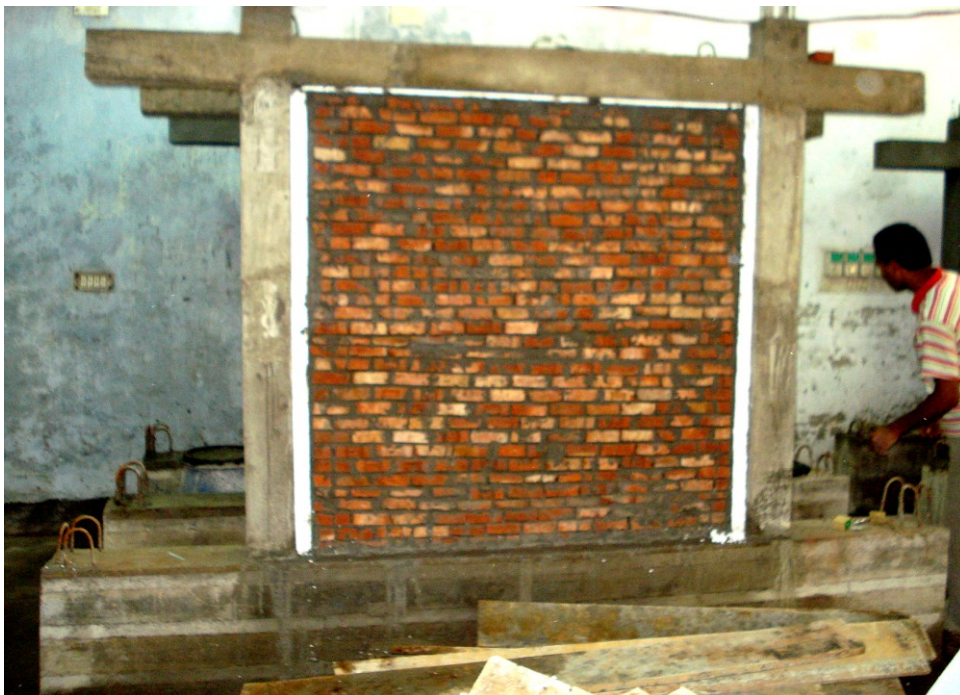
Figure 3.18 Application of cork sheets into gaps between the infill and the surrounding RC frame for the isolated infilled RC frame
