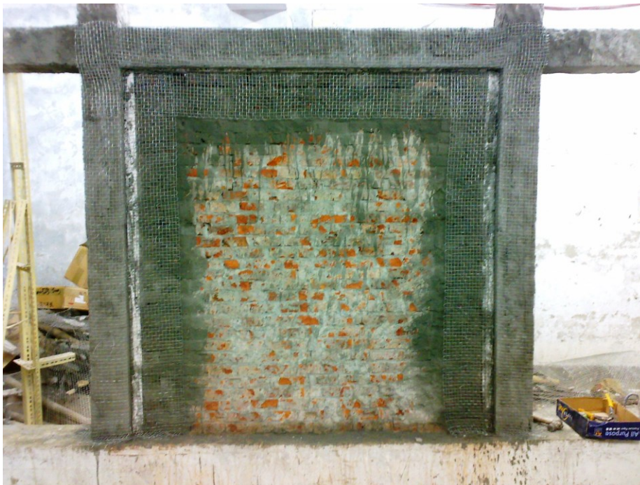
Figure 3.29(b) Gouting along the wrapped wiremesh around the RC frame and the infill RC frame interface
