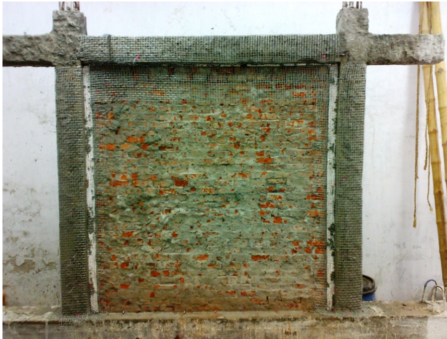
Figure 3.29(a) Wrapping of wiremesh on isolated infilled RC frame to repair the bed joint failures of isolated infill wall
