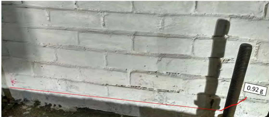
Figure 4.5 Horizontal Cracks develop at 0.92g (south wall)
