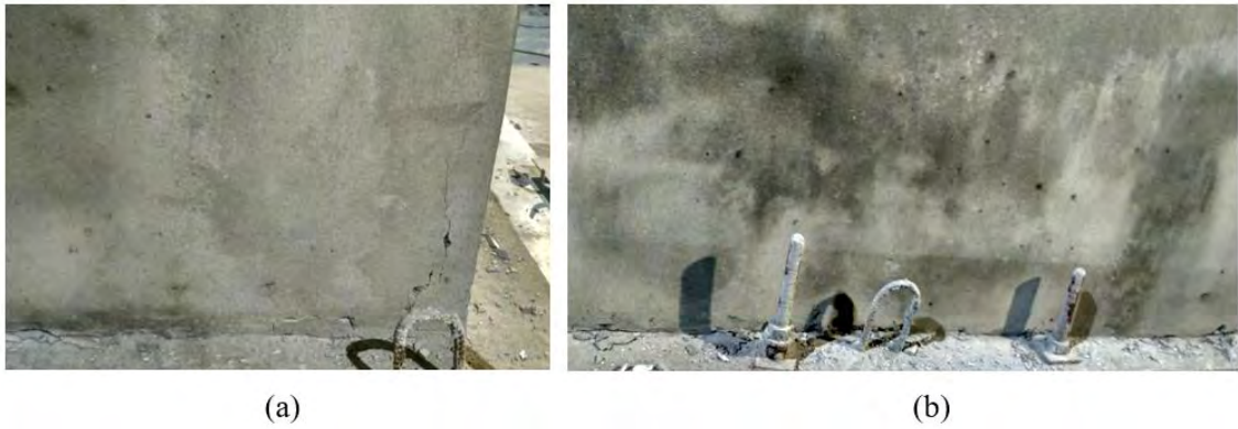
Figure 4.10 Crack developed in Retrofitted Model ((a) vertical crack in north wall (b) separation of wall from base)
