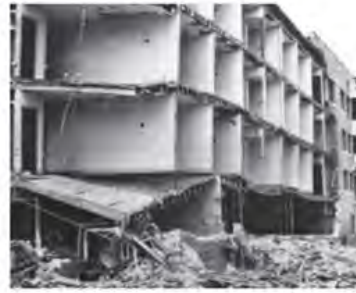
b) Heavily damaged Hotel Californian, 1925 Santa Barbara, California earthquake.
