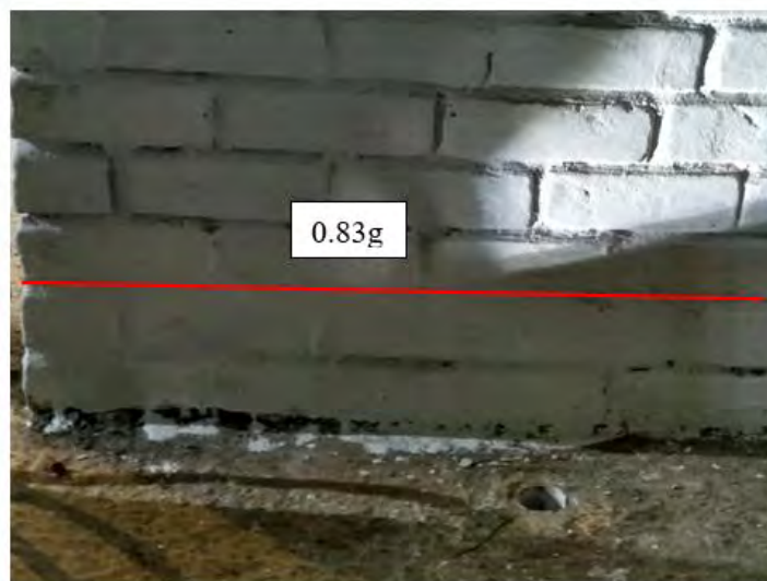
Figure 4.3 First crack develop at 0.83g in east wall (out of plane wall)
