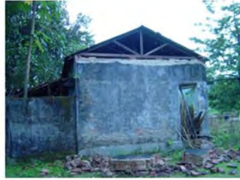
b) Damage due to 2003 Rangamati Earthquake
