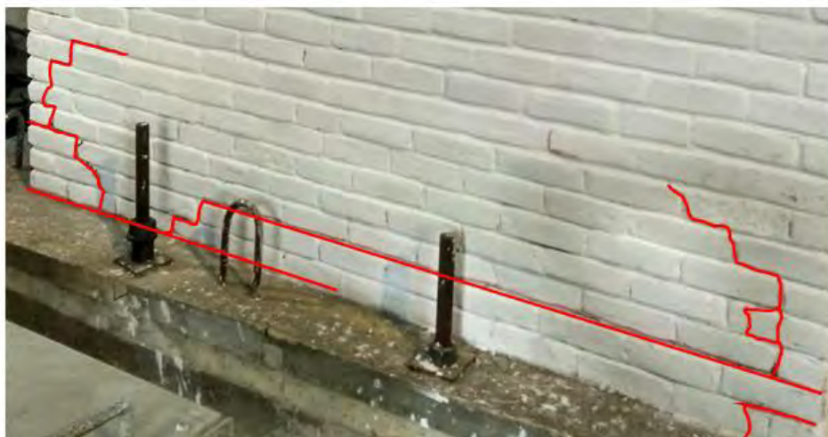
Figure 4.9 Cracks developed at 1.05g in west wall (out of plane wall)
