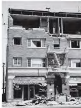
c) URM building damage, 1933 Long Beach, California earthquake
