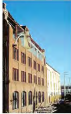
d) Upper story wall collapse, with resulting fatalities
