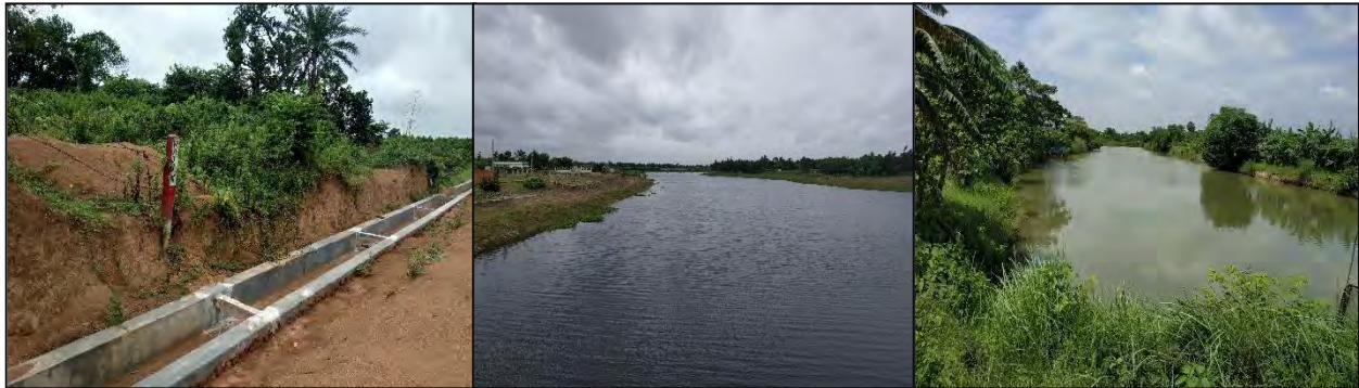
Figure 4.10: Drainage network alongside the road, Photo Taken on July 23, 2018
