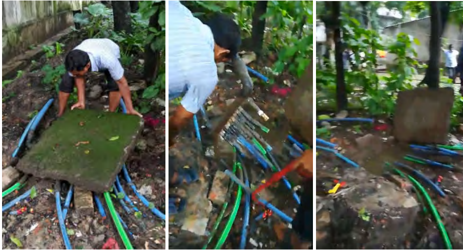
Figure 3.10: Illegal connections in DMA 507
