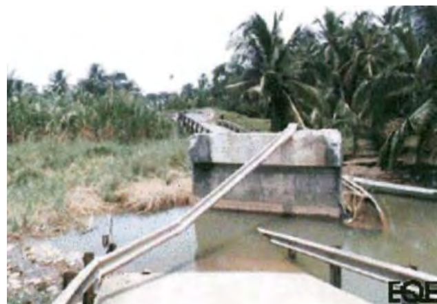
Figure 2.23: Unseating of Rio Bananito bridge in 1991 Costa Rica earthquake
