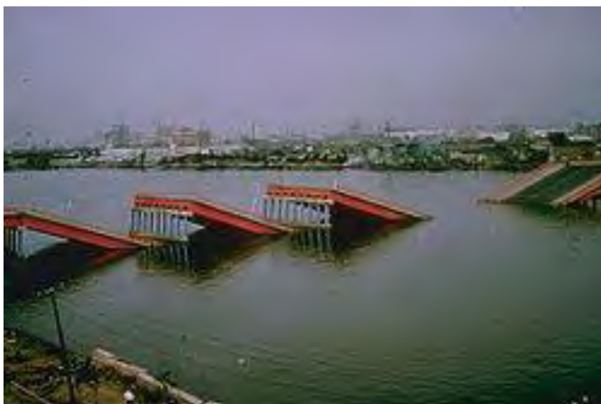
Figure 2.19: Damage to Showa bridge (Niigata earthquake, 1964)
