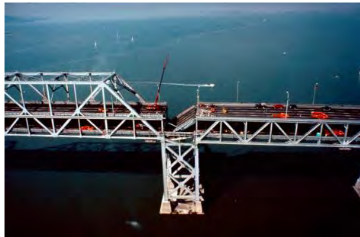
Figure 2.22: Oakland Bay bridge damaged by Lorna Prieta earthquake (EERI, 1990)
