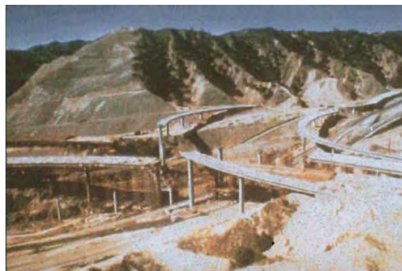
Figure 2.20: Span collapse (San Fernando earthquake, 1971)
