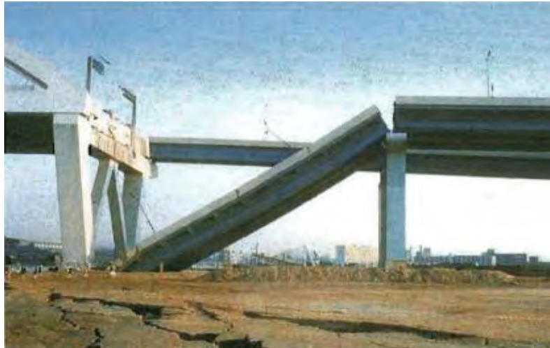
Figure 2.25: Unseating of Nishinomiya-ko bridge in Kobe earthquake (1995)
