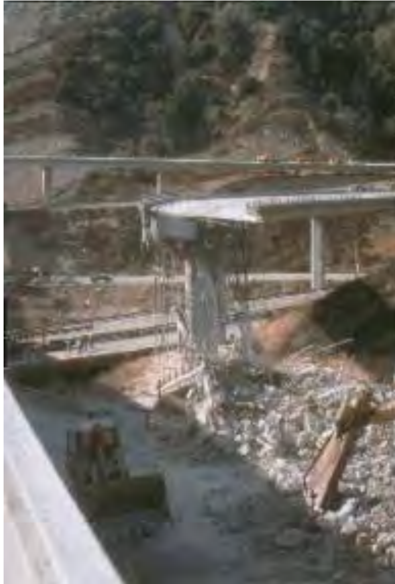
Figure 2.24: Damage due to Northridge earthquake
