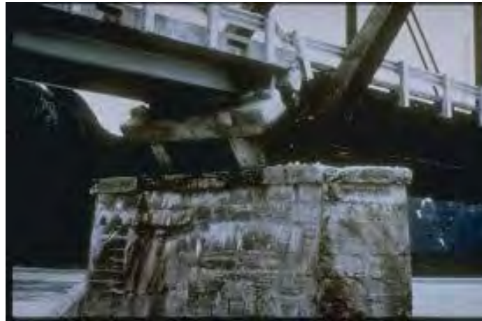
Figure 2.18: Damage to railroad bridges (Alaska earthquake, 1964)
