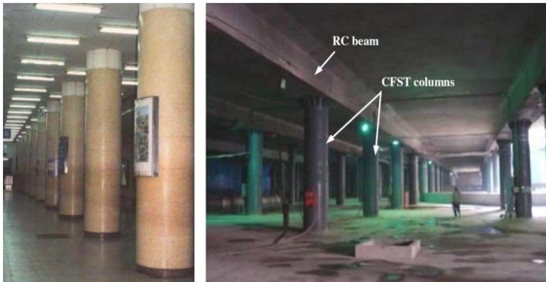
Figure 2.4 CFST columns used in a subway station.
