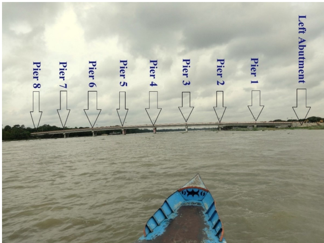
Photo 3.2: Photo taken from the downstream of the bridge displaying its piers, deck and left abutment.
