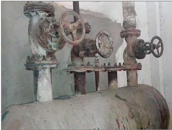
Un-insulated Steam Header and valves
