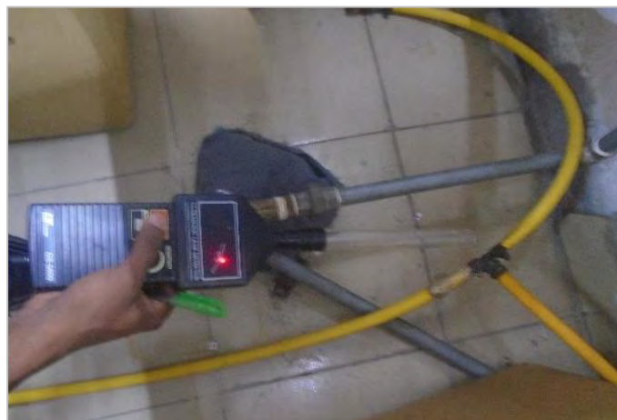
Figure 4.13: Air Leakage Found During Compressed Air Leak Test
