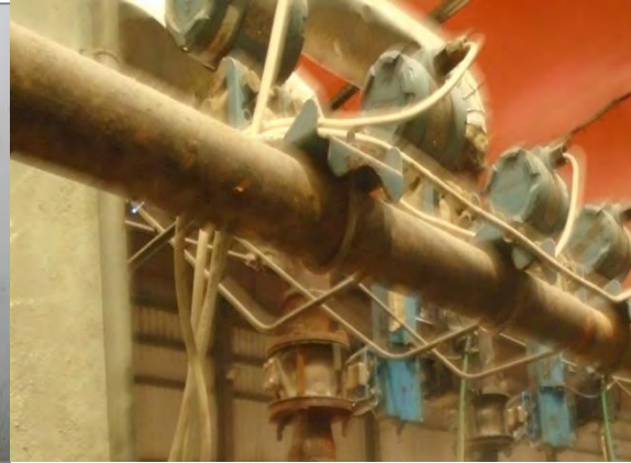
Un-insulated Steam Line
