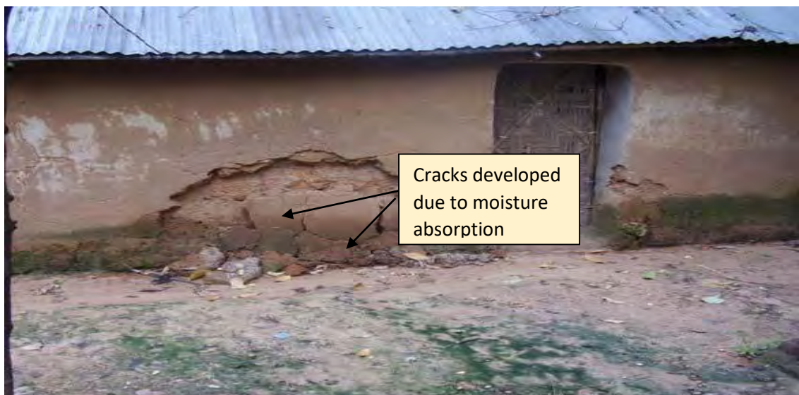
Fig. 2.11: Damage of wall due to moisture absorption
