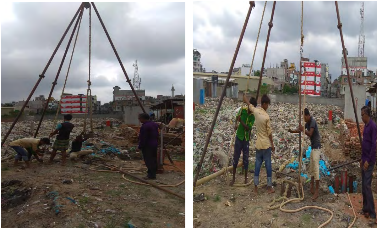
Figure 3.4: Percussion drilling of the borehole where the tests were carried out as at the time of ground water sample collection.
