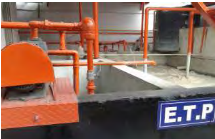
Figure 3.3: Effluent Treatment Plant(ETP) of a renowned Pharmaceutical Industry.
