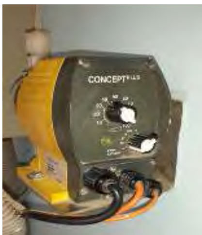
Figure 3.6: NaOH dosing pump of decontamination unit
