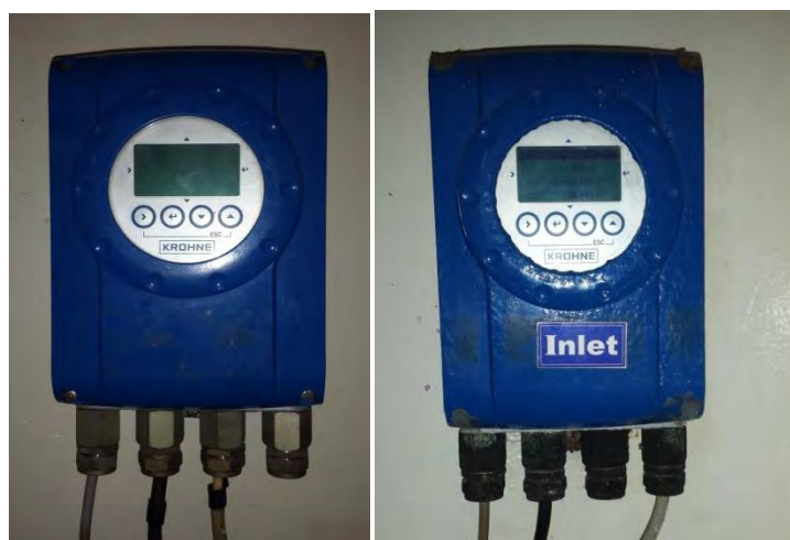
(a) Flow Meter used in Decontamination Tank
