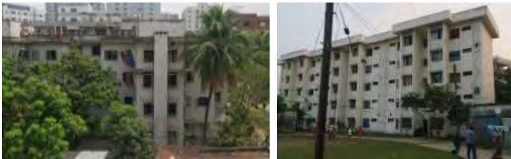
Fig 2.2: Walk up House type; Green road government housing (left), Mirpur BCSIR staff housing (right)
