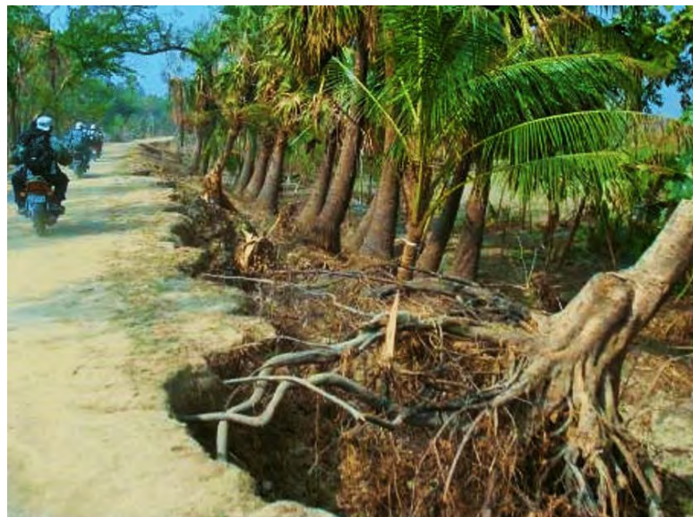
Figure 2.15: Failure of Embankment due to Overturning or Uprooting of Trees during Cyclone (Mohammad Shariful Islam, BUET)
