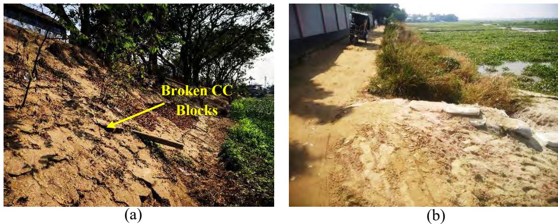
Figure 4.24: Photographs of Protection Type III; (a) Kalikaccha, Sarail, Brahmanbaria; and (b) Modhupur, Ashuganj, Brahmanbaria
