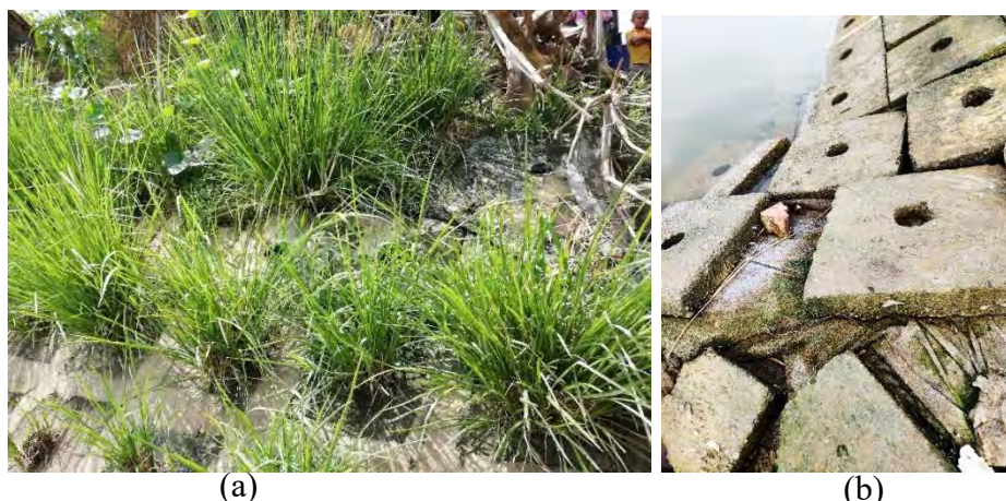
Figure 4.29: Photographs of Protection Type III; (a) Meghna Natunpara, Derai, Sunamganj; and (b) Kachua, Derai, Sunamganj
