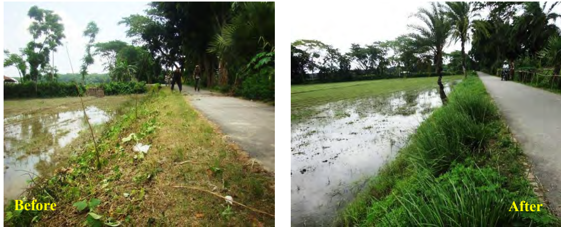
Figure 2.22: Road Slope Protection by Vetiver at Barisal, Bangladesh under CCRIP (Islam and Hoque, 2020)
