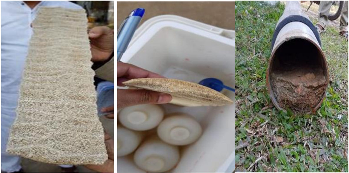
Figure 2.4: Scaling in pipes at Meherpur WTP [7]
