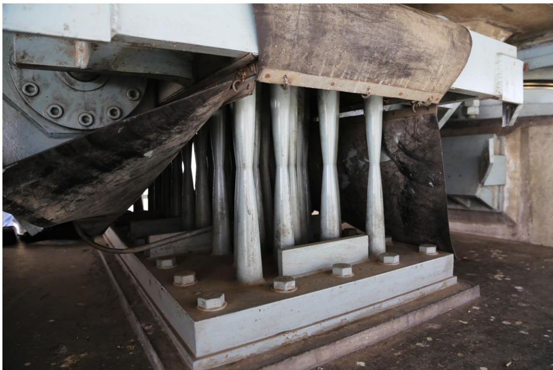
Fig. 2.34: Pintle damper in the Bangabandhu Bridge
