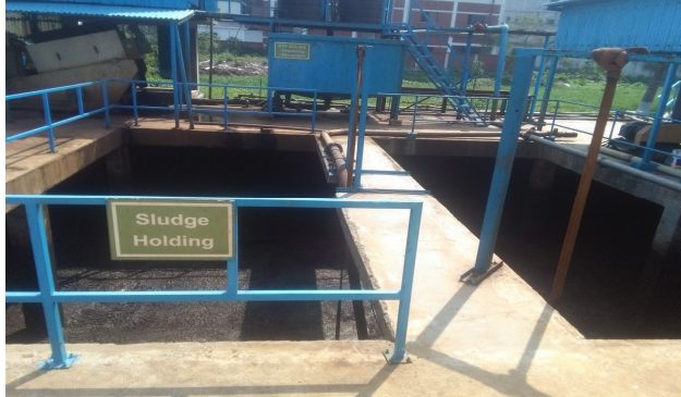
Fig. 2.8 Sludge thickening tank
