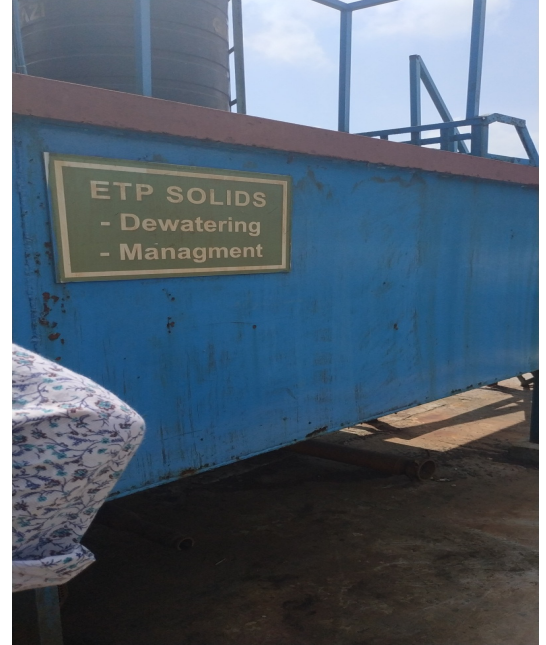
Fig.2.10 Sludge dewatering machine
