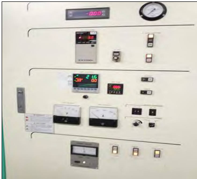
Figure-3.4: Control panel of SPS machine
