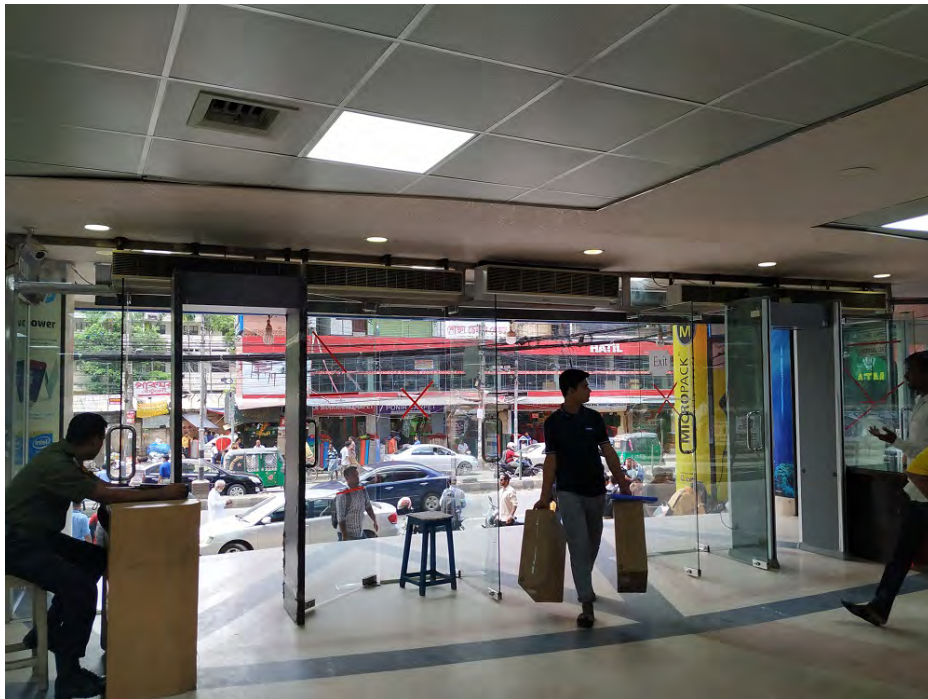
Fig. 1.17 Photographs of already installed air curtains in mall entrance at MultiPlan Shopping Complex of New Elephant Road, during the survey.
