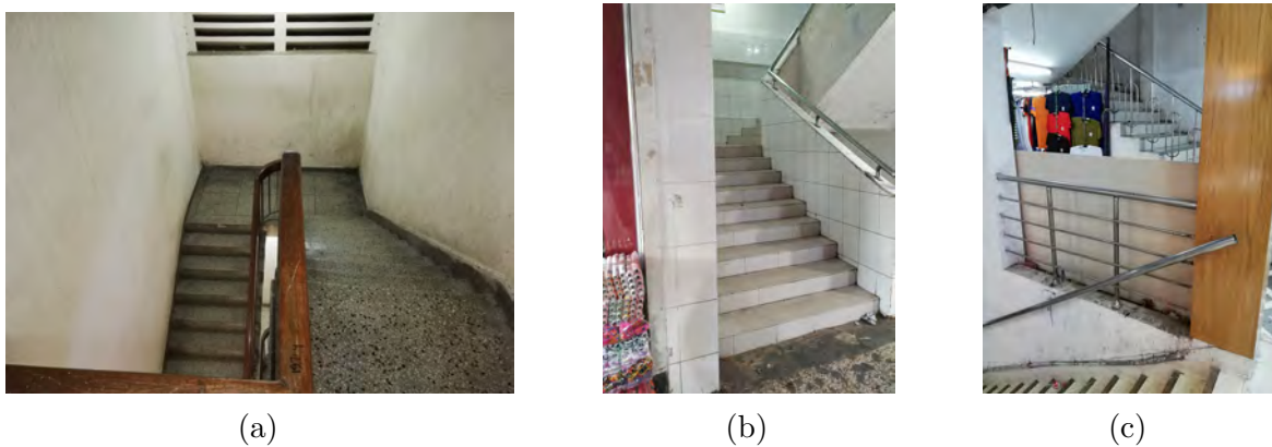
Fig. 1.12 Photographed staircase of (a) UAE Maitry complex, (b) Muktijoddha market, and (c) Nurjahan Supermarket during the survey.
