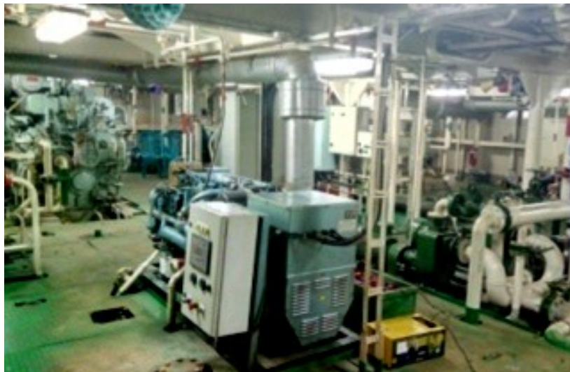
Fig. 5.9: Machinery items inside the engine room of an inland passenger ship, source: author.
