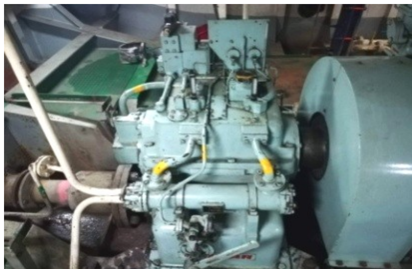
Fig. 5.10: Accumulation of spilled oil under the machinery items inside the engine room, source: author.
