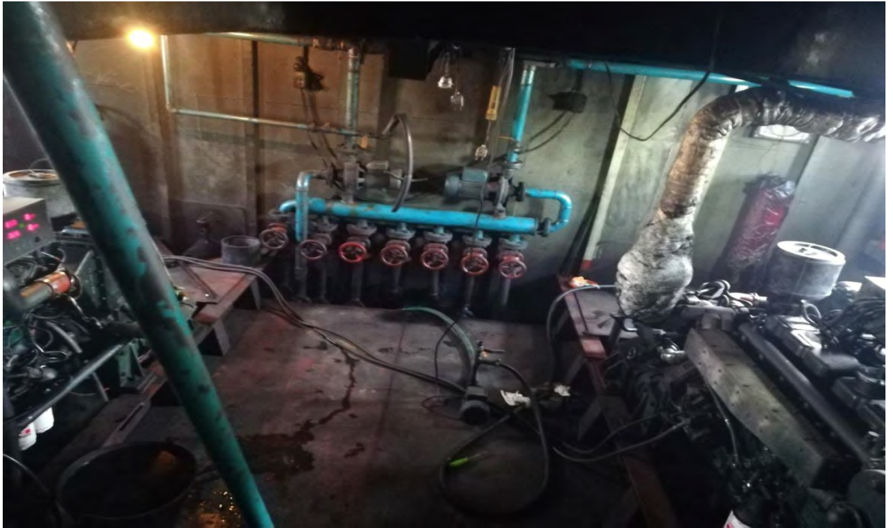
Figure A-D.9: Water Bus Engine Room
