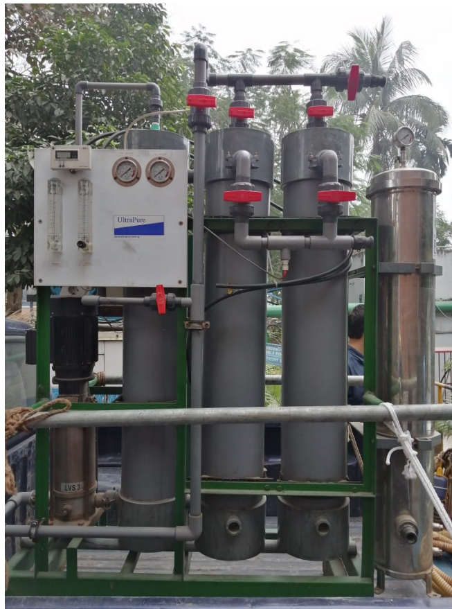
Figure 3.1: Setup of the mobile filtration unit
