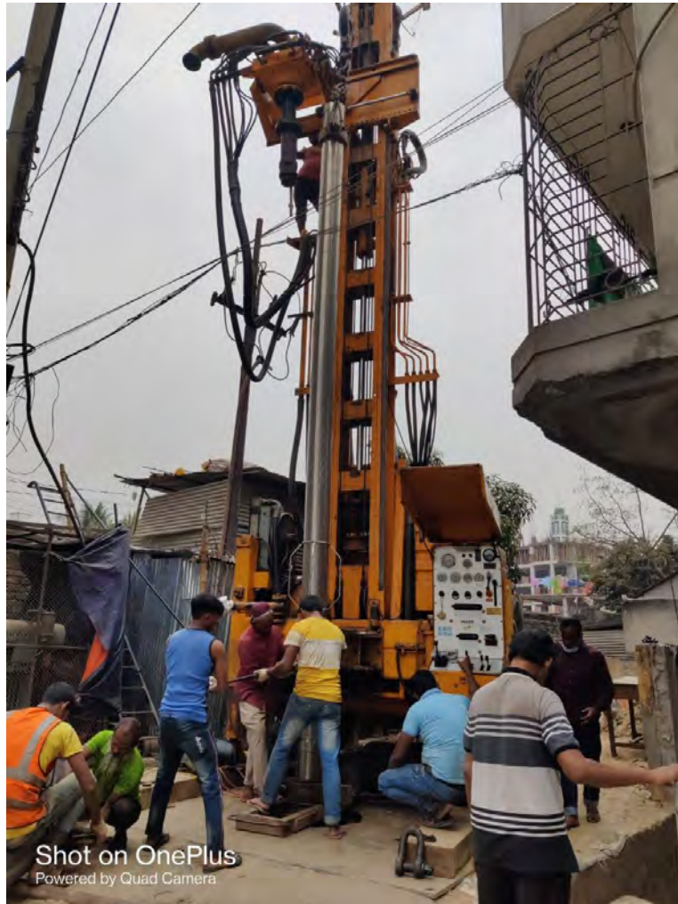
Photo 6.3: View of Boring for Installation of a New Deep Tubewell (Photo taken on 8 March, 2021)
