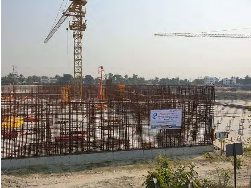
Photo 6.1: Construction Site of Gandharbpur Surface Water Treatment Plant Phase- I (Photo taken on 2 February, 2021).
