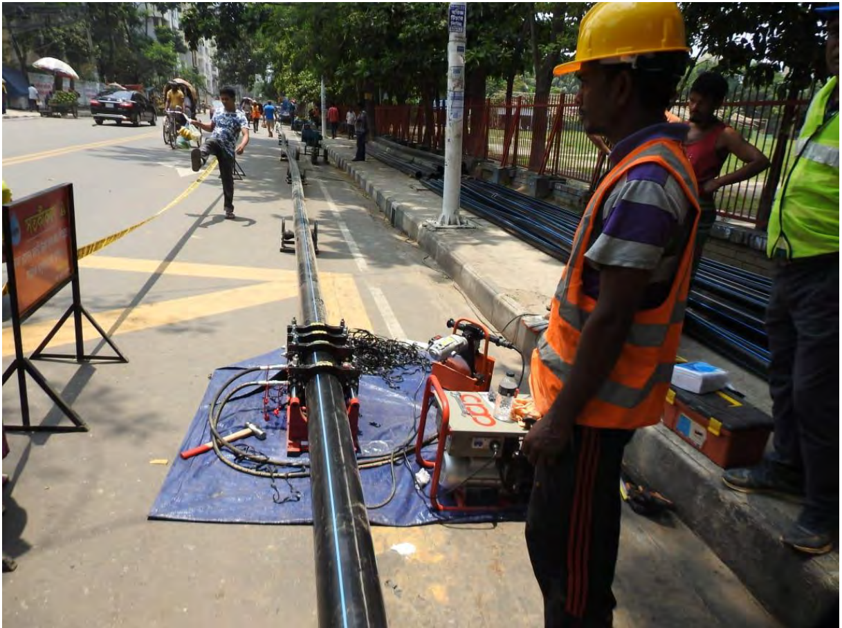
Photo 6.4: Construction of a New DMA by Replacing the Old Pipes with the HDPE Pipes
