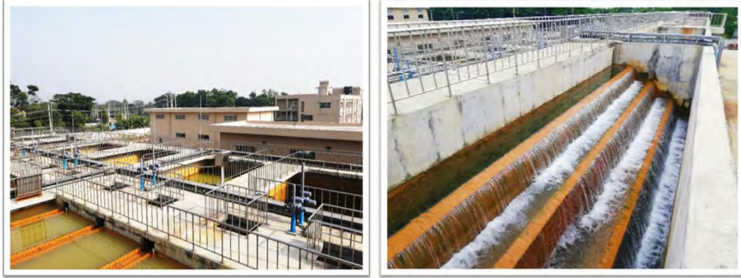
Photo 6.2: Tetuljhora - Bhakurta Well Field with Iron Removal Plant (Photo taken on 13 February,2021)
