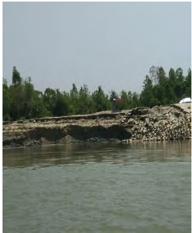
Figure 5.66: Failure of protection works during recession time of floodwater.
