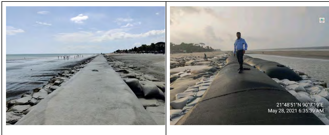
Figure 1.7: Protection by geo-tube and geo-bag to combat erosion in Kuakata beach (Photograph Courtesy: Engr. M.H Salehy, EXEN, BWDB; May 28,2021)
