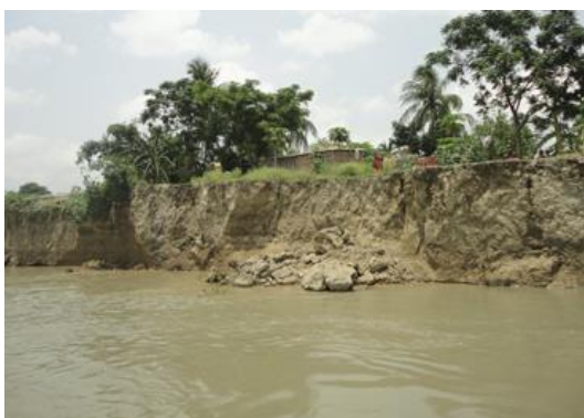
Figure 4-4: River erosion caused loss of lands along Padma River (Source: google)
