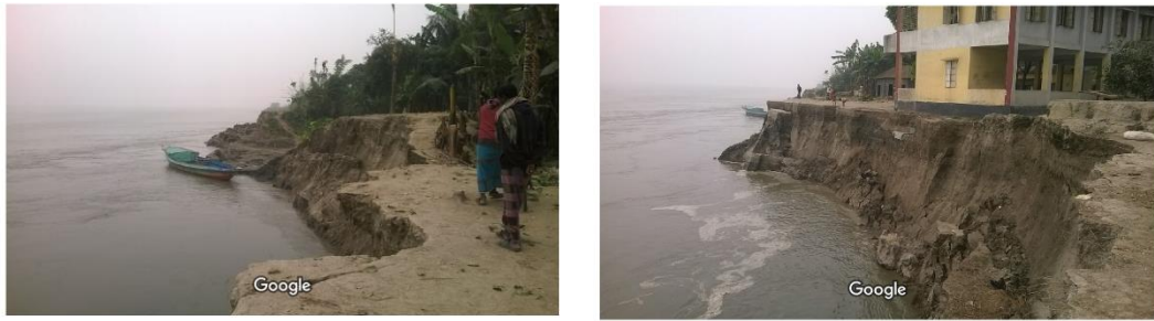
Figure 4-9: Erosion along the Padma River Bank in Harirampur (Source: google)
