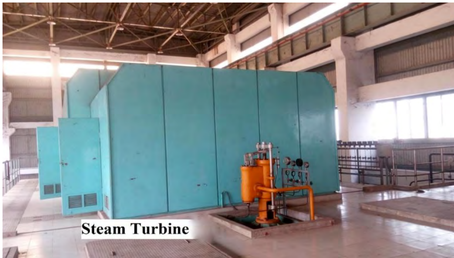
Figure 3.7: Steam Turbine Hall.
