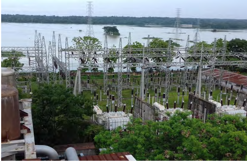
Figure 3.13: 132 kV substation yard.
