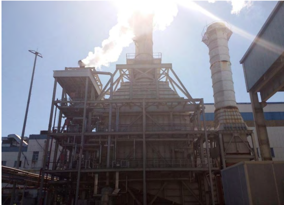
Figure 3.6: Heat recovery steam generator.
