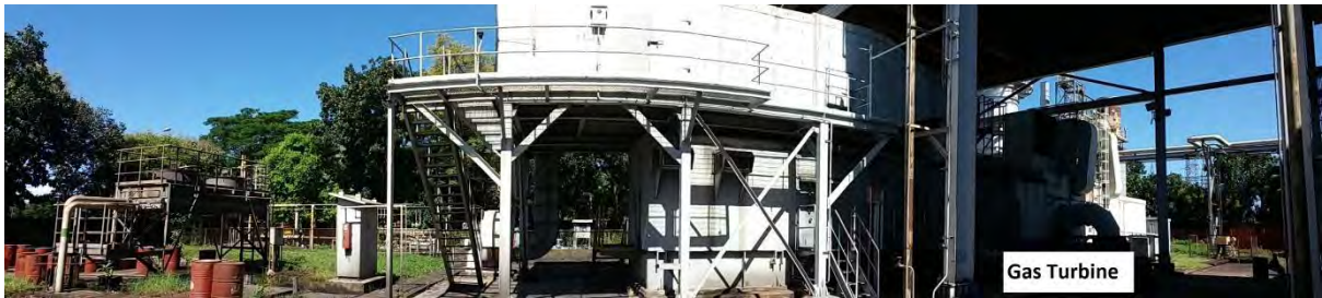
Figure 3.5: Gas Turbine Unit side view.
