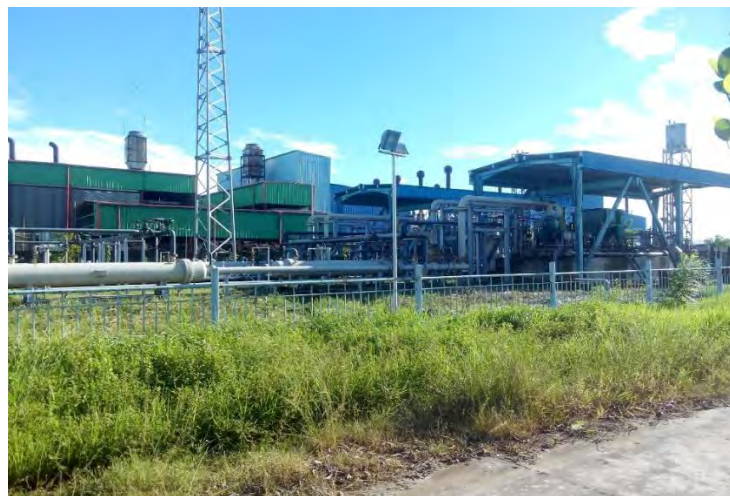
Figure 3.12: Gas booster Unit.
