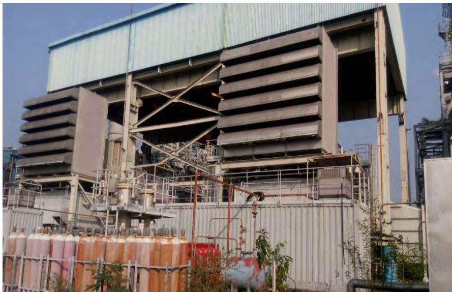
Figure 3.4: Gas Turbine Unit
