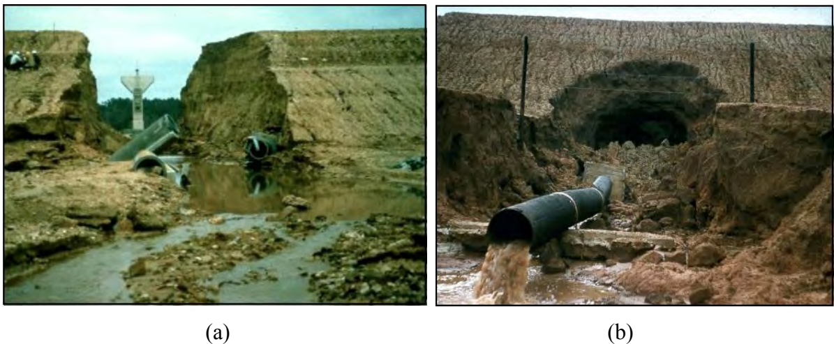
Figure 2.4: (a) Washed away embankment, (b) piping failure of embankment constructed on dispersive soil (Mississippi, USA) (source: www.fema.gov )
