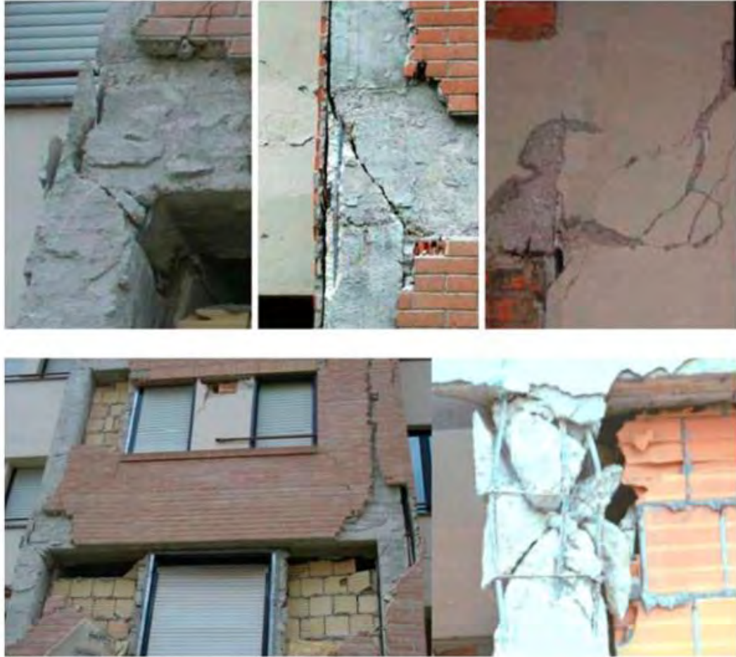
Figure 2.22: Effects of local infill–frame interaction: Sample of the local shear collapse of column ends and joints due to the interaction with the infills (Trapani et al., 2015).
