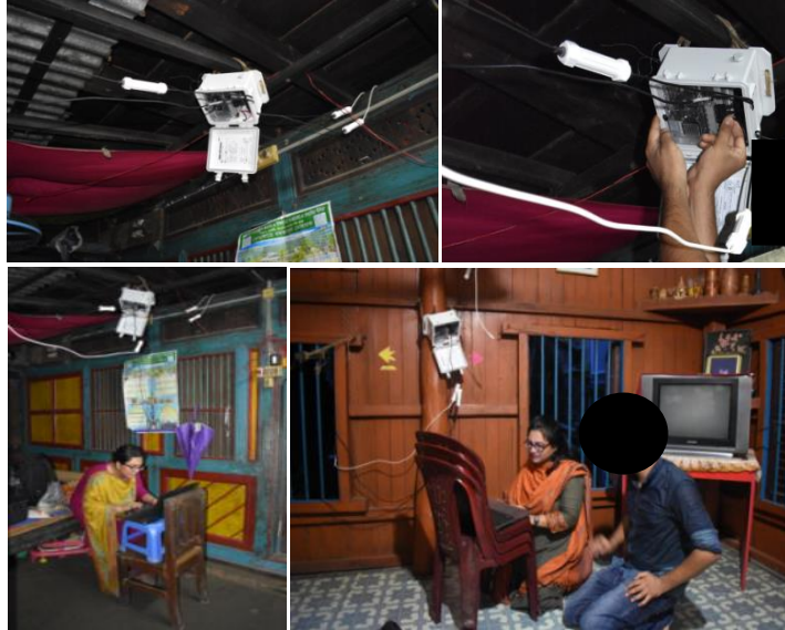
Figure 3.2 Data logger installation at traditional timber houses
