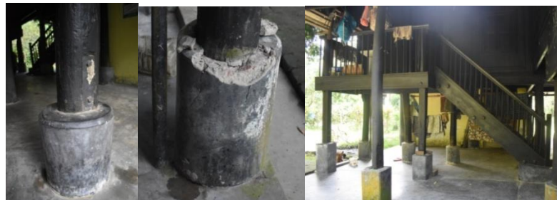
Figure 4.19 Concrete base under the stilts for protection from ground moisture and flood-water
