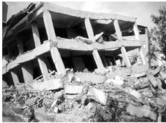
Fig.1.1: Exterior joint failure during the 1999 Kocaeli Turkey earthquake (Ghobarah and Said, 2002)
