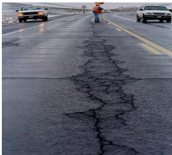
Figure 2.14: Fatigue cracking caused by stripping.
