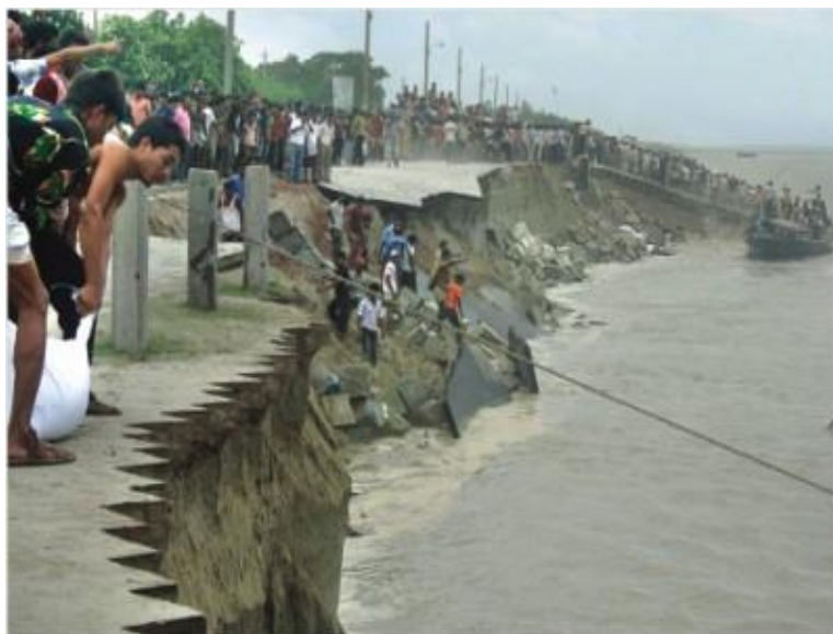
Figure 2.6: Modes of failure of Sirajganj Hardpoint at 2009.
