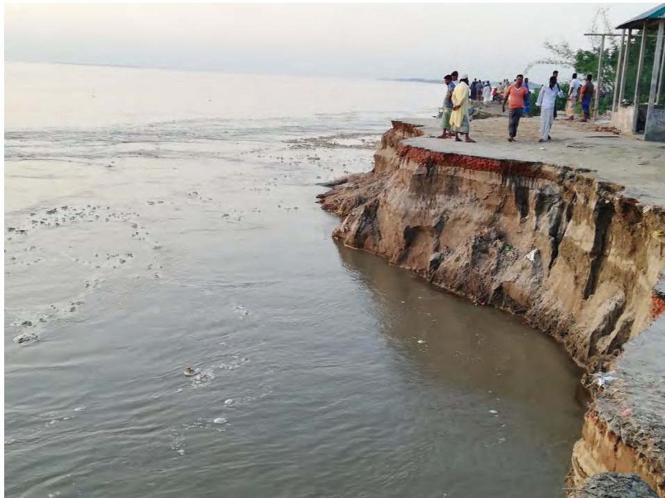
Figure C 8: Eroded LGED road in Attached Char
