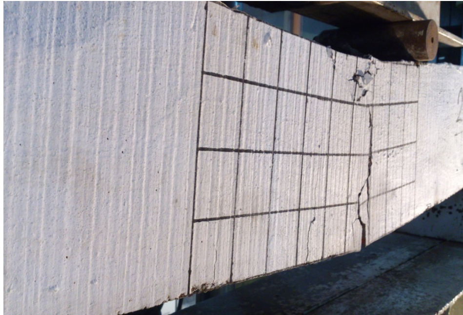
Figure 5.47: Crack-pattern for 2.5% GWRC specimen
