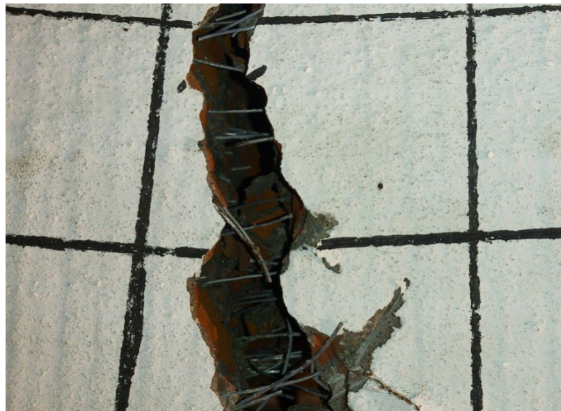
Figure 5.38: GI wire fibers spanning across the crack
