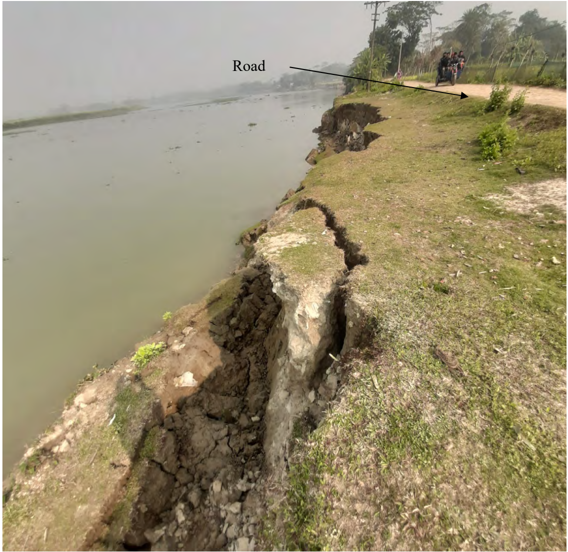
Photo D13: View showing massive erosion adjacent to the brick-soling road at the bend 22.
