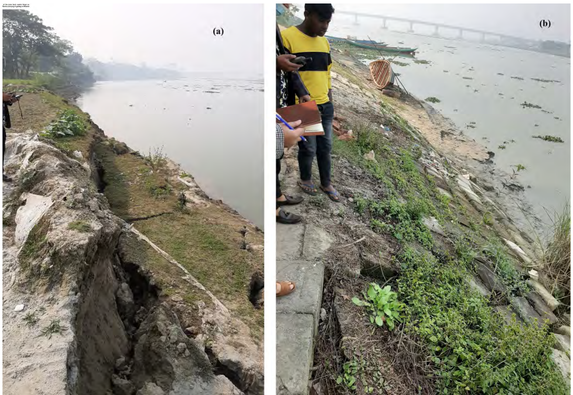
Photo D12: Photos represent the inspection of unprotected and protected banks of bend B22 at Khasherhat Bazar at Kalkini Upazila, Madaripur. Left photo - erosion by mass failure, right photo-Khasherhat Bondor protection project.
