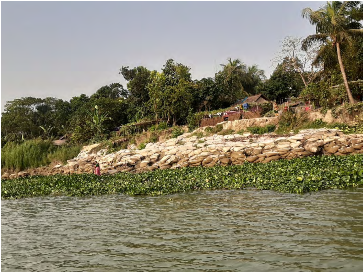
Photo D10: Photo showing ineffective temporary river protection- unplanned dumping of geobag at erosion prone bank.
