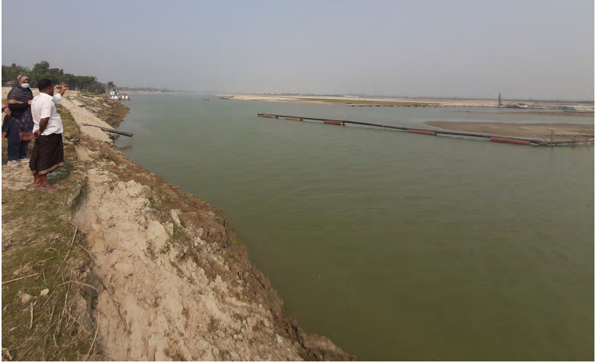
Photo D5: View of river navigation improvement by dredging project at the upper reach of the Arial Khan River.
